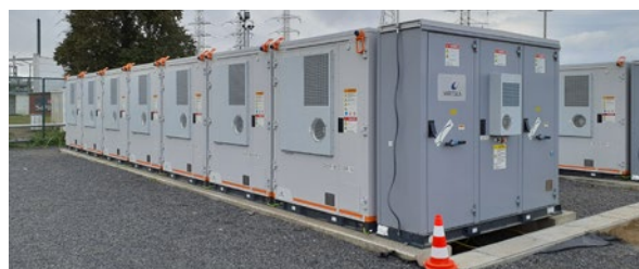
Ruien Power Storage Station in Belgium
