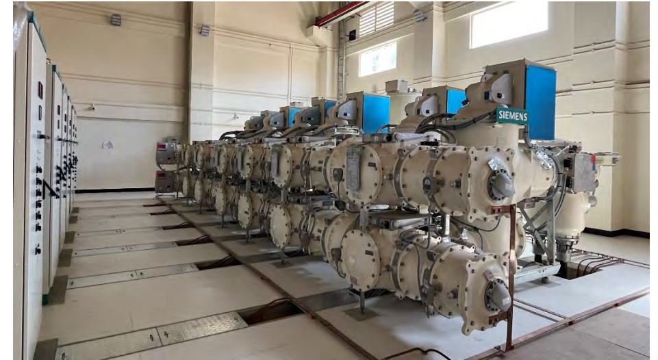
Inside the substation building
