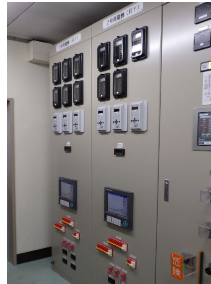
The power generator control equipment delivered
