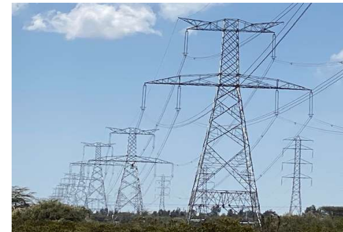
400 kV transmission line
