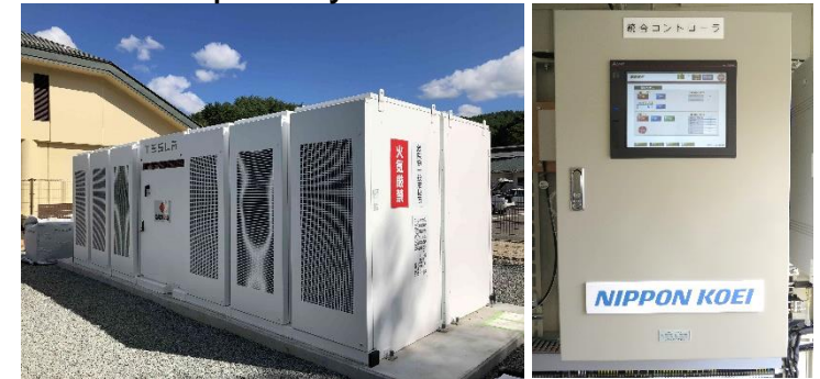
Battery storage system, exterior of the local EMS equipment
