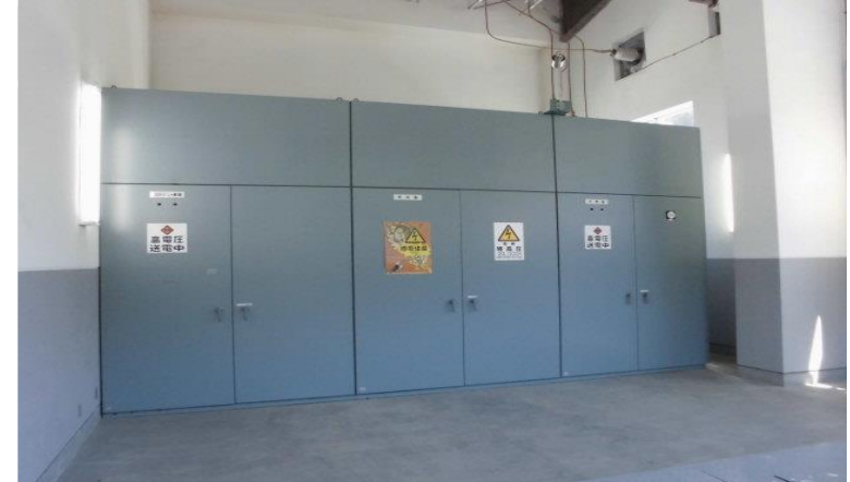
30 kV switching equipment
