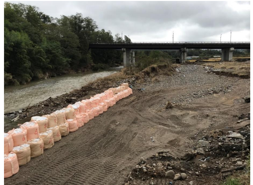
Location of the collapsed levee of the Namezu River, the branch river of the Chikuma River
