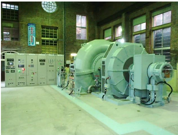
Water turbine generator control system
