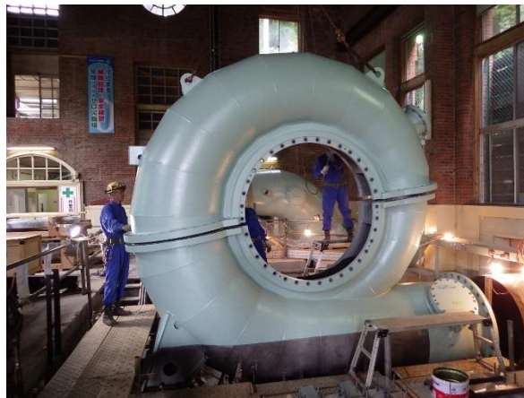
Water turbine assembly
