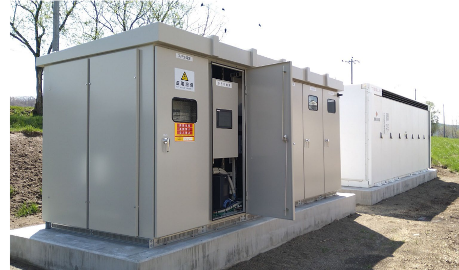
EMS and power storage system
