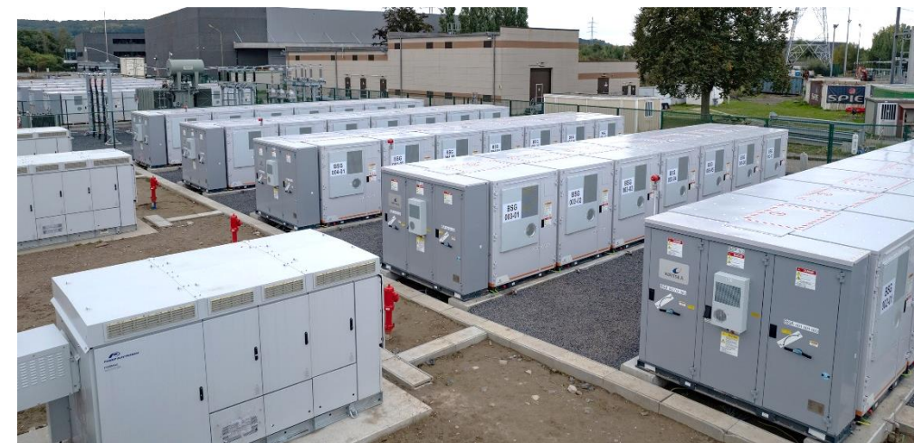
Battery-based energy storage system in Ruien, Belgium
