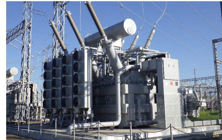
No.6 transformer (275kV/154kV, 450MVA)
