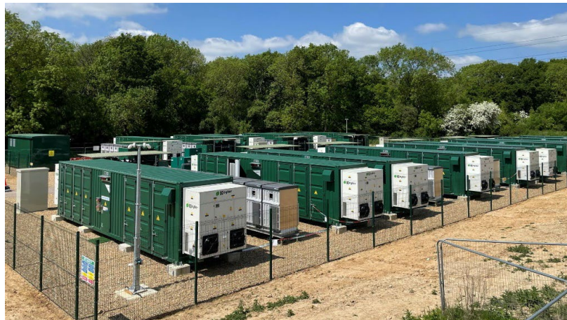
Panoramic view of the energy storage plant (49.5MW/49.5MWh)
