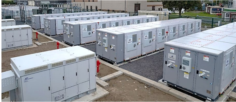
Battery storage station in Ruien, Belgium
