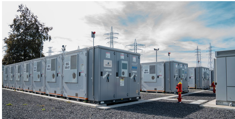
Ruien Energy Storage
