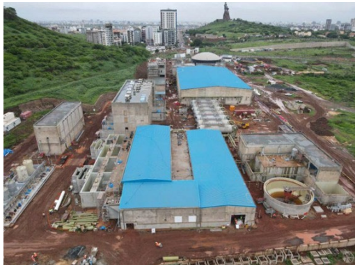
Overall view of the plant
