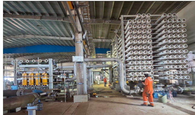
Inside the RO (reverse osmosis: membrane process technology that removes salt from seawater) building
