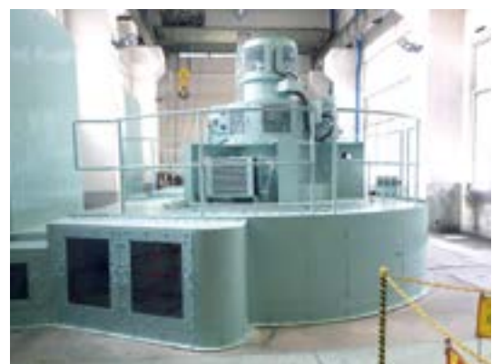
Vertical synchronous generator
