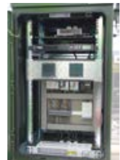
Storage battery control system
