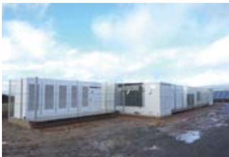
Full view of the 4 MW storage battery
