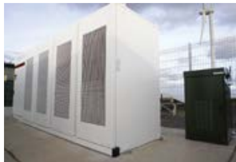
4-MW rechargeable battery (left), Storage battery control system (right)
