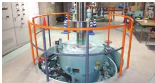
Vertical Francis turbine
