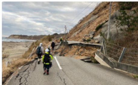
Field survey after the earthquake
