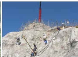
Construction work with rope access technicians, the first of its kind in Nepal
