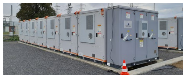
Ruien Power Storage Station in Belgium
