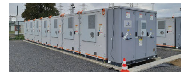
Ruien Power Storage Station in Belgium
